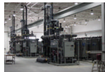
Carlton Treatment Plant
